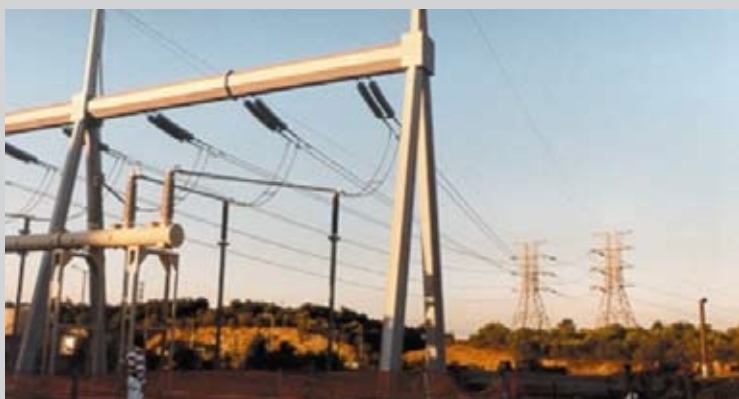
132kV transmission Channel Island, Northern Territory.
