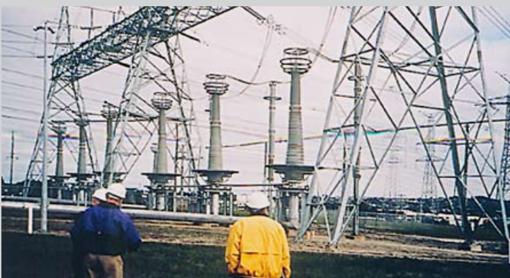
Rowville 500kV terminal station, Victoria.
