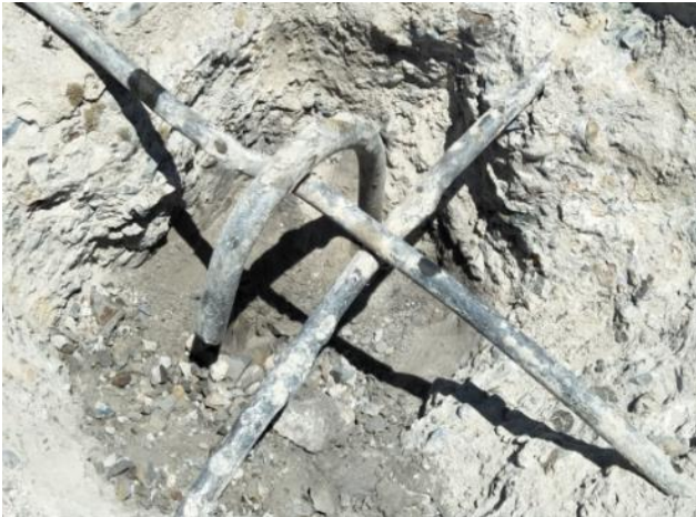
Figure 3 - Condition of existing reinforcement
