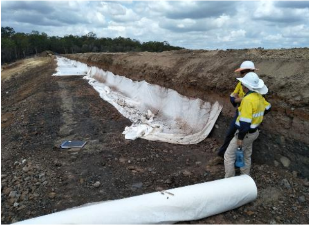
Figure 10 - Granular materials uncovered at crest
